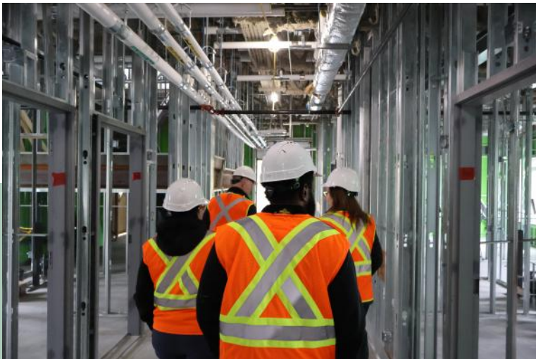
The DRDH Team walking through a resident wing with completed interior framing.
