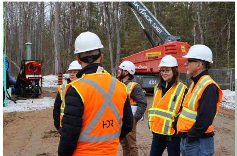
President & CEO Janna Hotson and Board Vice Chair Christian Kaiser inspecting exterior progress.
