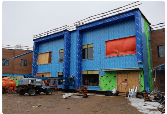
Enclosure is nearing completion on the main entrance to the Four Seasons Lodge LTC Home
