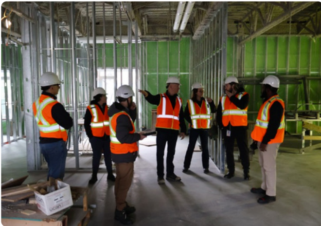
The DRDH Team discussing uses of communal spaces in the new Four Seasons Lodge LTC Home
