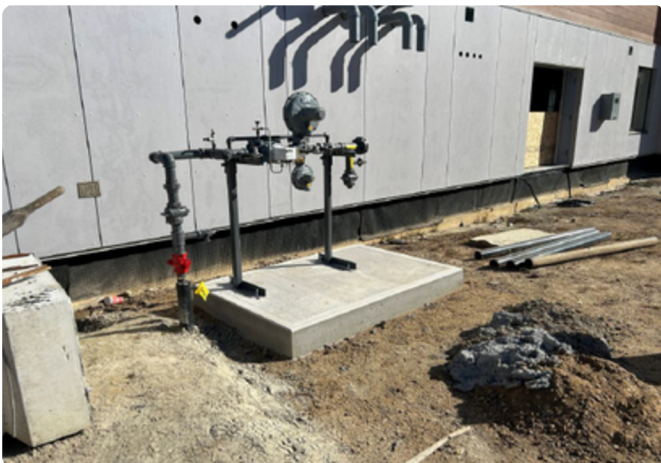
View of Enbridge gas supply meter in place on concrete pad.
